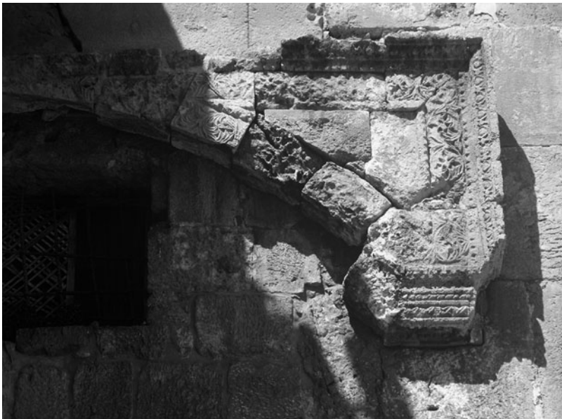
Fig. 9.5. An Umayyad decorative addition to the western Huldah Gate. Photo H. Bloedhorn.
